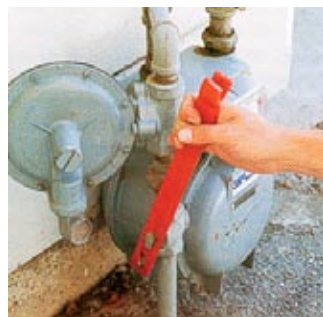
Gas. Shut off gas at the meter only if you suspect a leak.
