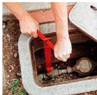
Water. If your water lines are broken, shut off water at the main valve at the street.
